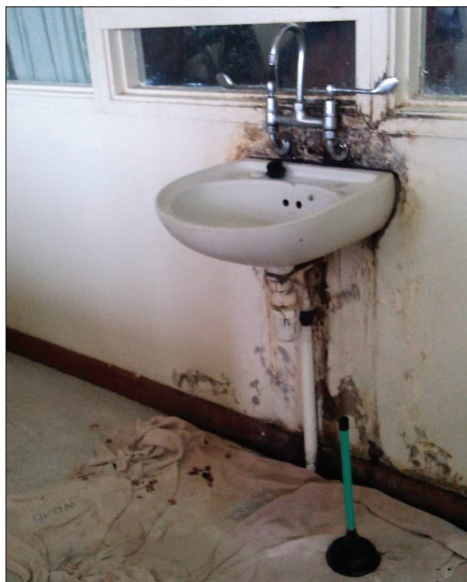
Figure 2. The sink in an isolation room for immunocompromised children.
